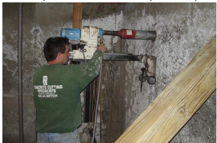
An engineer removes a core sample from a Connecticut home where the pyrrhotite-tainted concrete foundation was found to be cracking. Photo courtesy of Jim Okun
